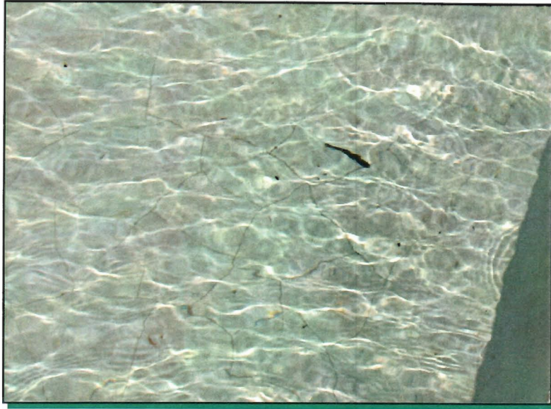
Cracked plaster finish at wading pool
