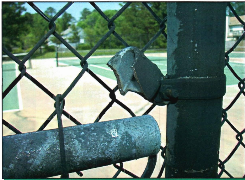
Damaged cross bar and connection of tennis court fence
