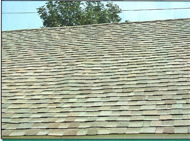
Sheathing deflection of asphalt shingle roof
