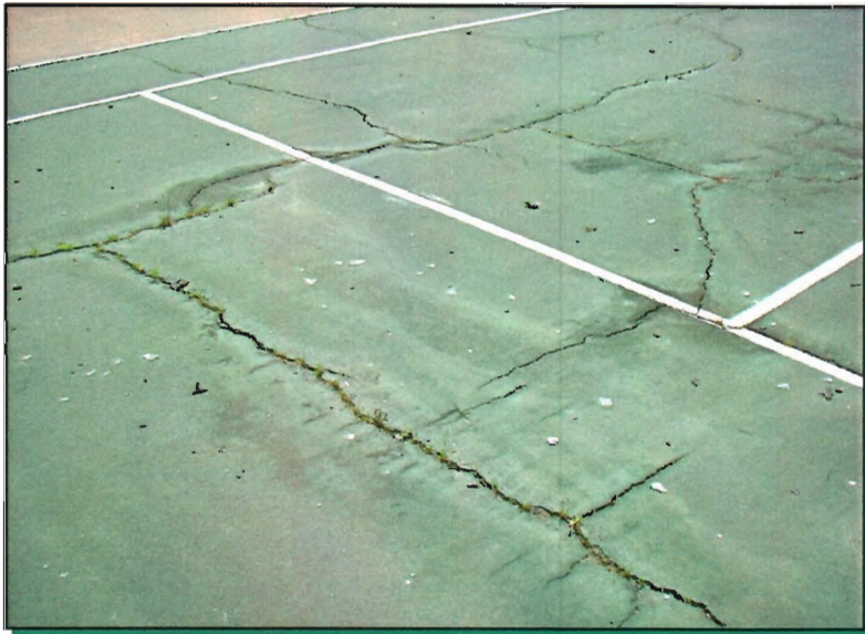
Cracked and organic growth through asphalt tennis court
