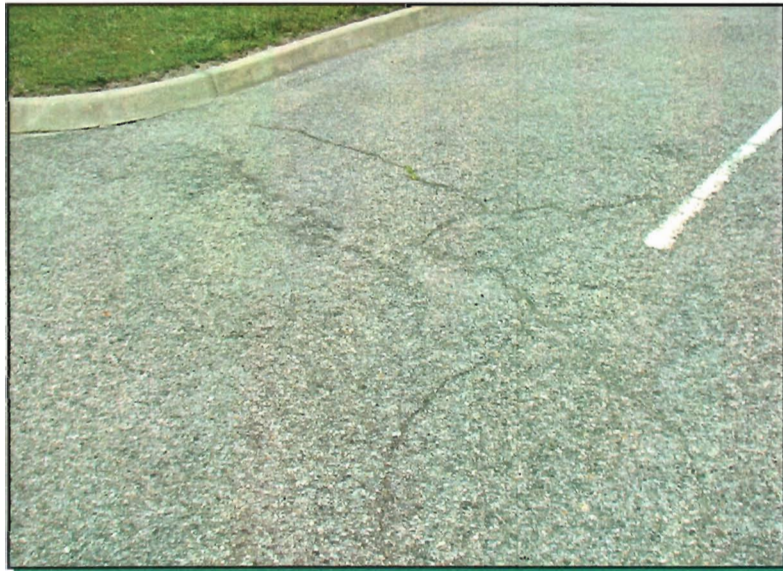
Cracked and surface raveled asphalt pavement
