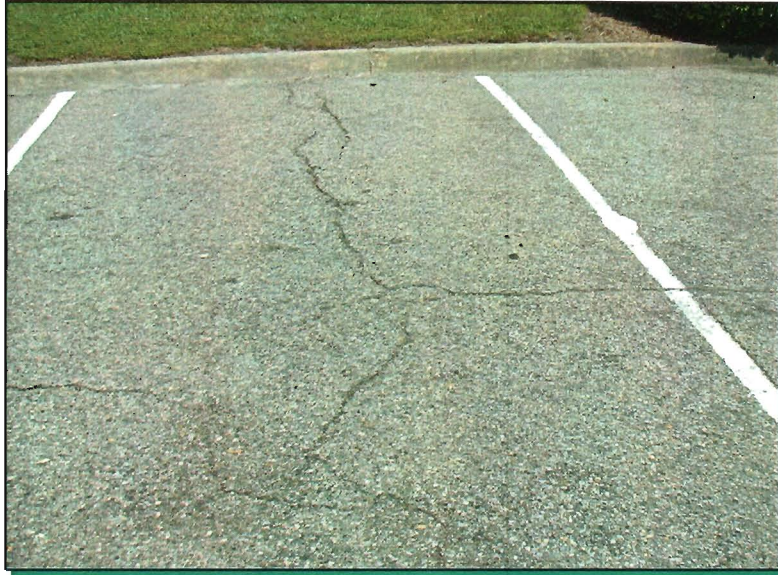
Cracked and surface raveled asphalt pavement
