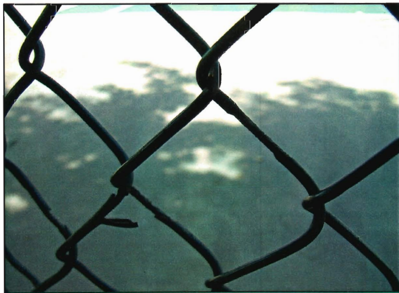
Damaged chain link section of tennis court fence
