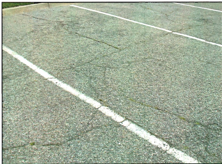
Cracked and surface raveled asphalt pavement
