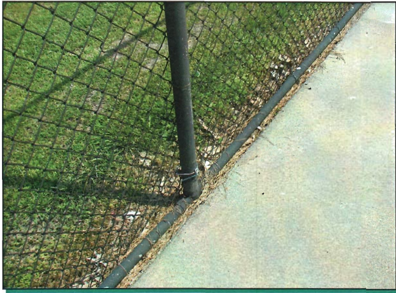
Damaged cross bar of pool fence
