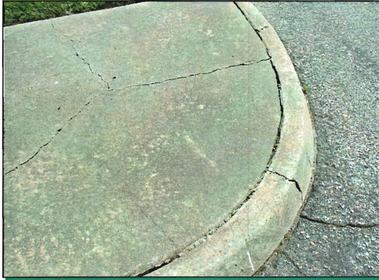
Cracked concrete sidewalk and curb, evidence of previous asphalt overlay
