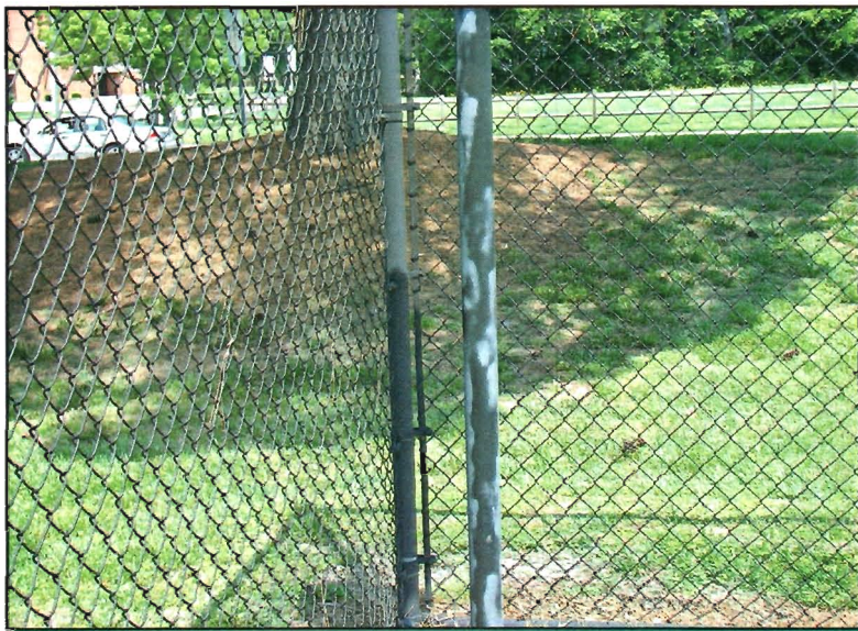
Deteriorated finish at light post
