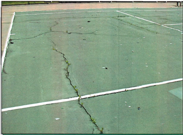
Cracked and organic growth through tennis court
