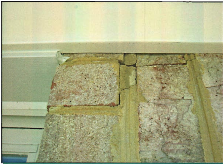
Deteriorated mortar - repair through the operation budget
