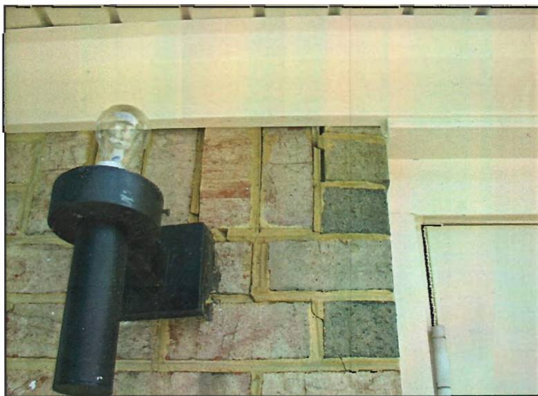
Damaged light fixture and deteriorated mortar- replace and repair through the operation budget
