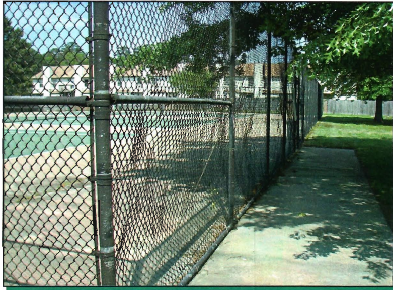
Tennis court fence - note damaged fence sections
