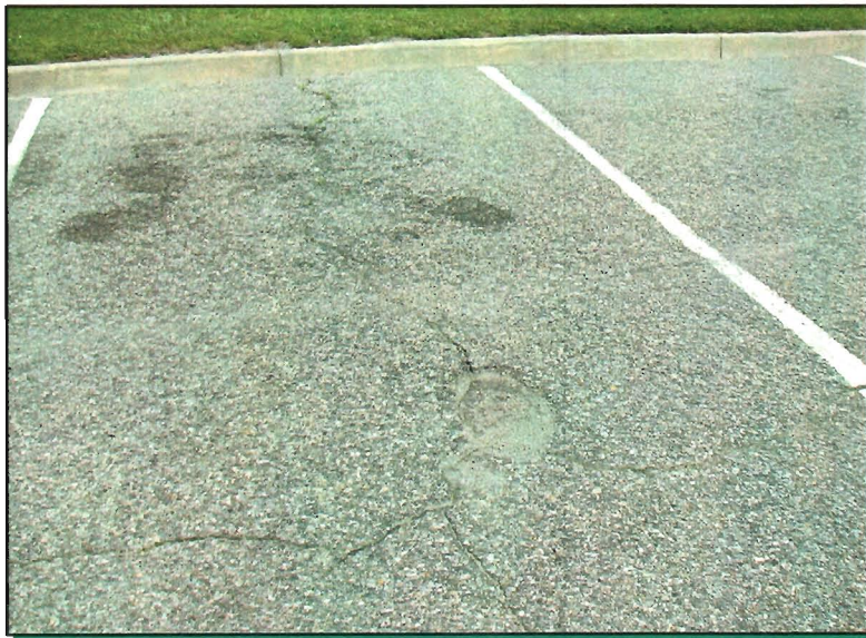
Cracked, surface raveled and evidence of a pothole at the asphalt pavement
