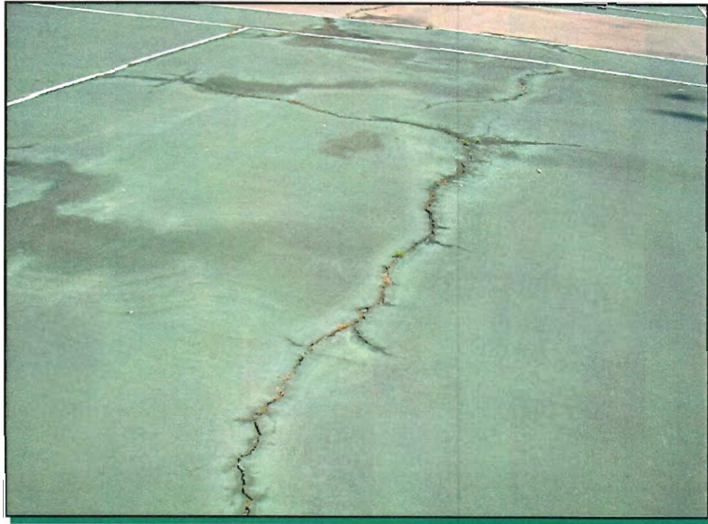
Cracked asphalt tennis court
