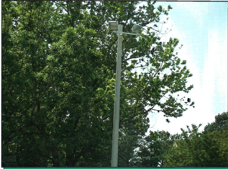
Light pole and fixtures
