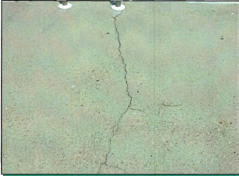
Cracked concrete deck
