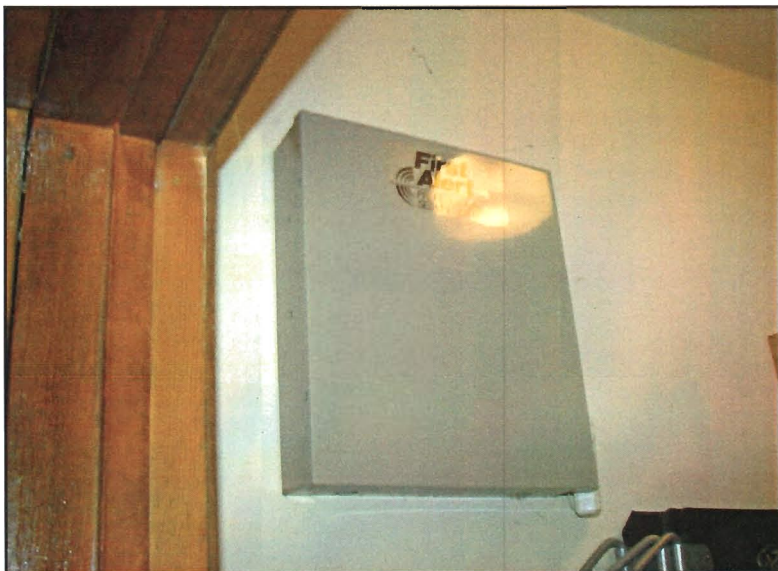
Security system control panel
