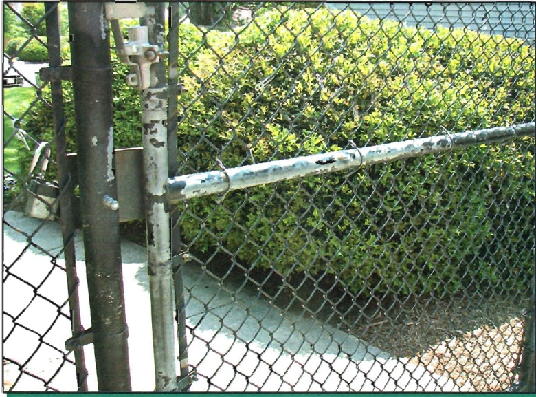
Finish deterioration of pool fence
