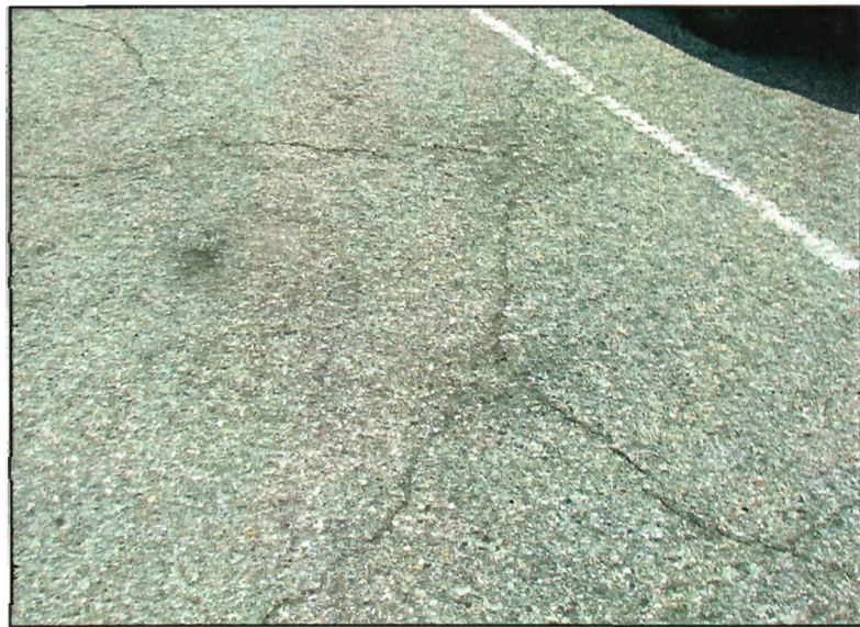
Cracked and surface raveled asphalt pavement
