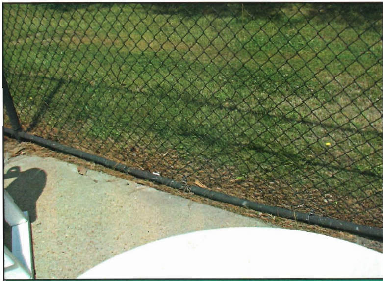
Damaged cross bar of pool fence
