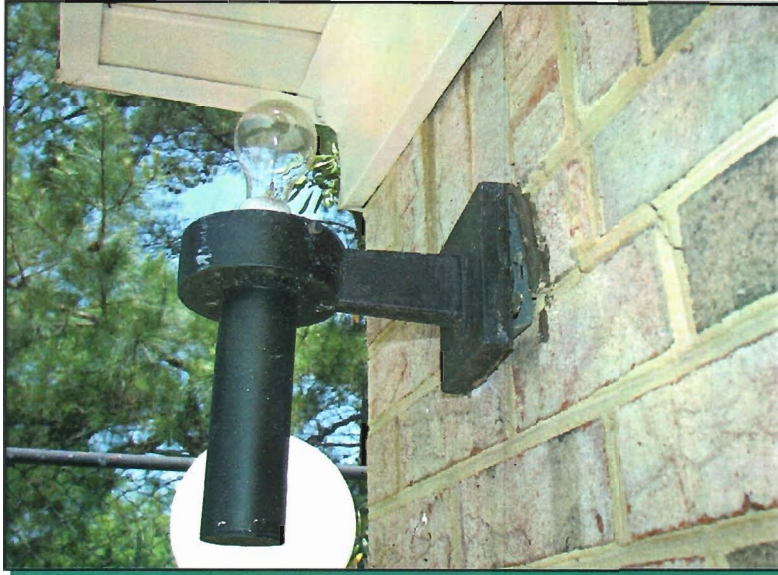
Damaged light fixture - replace through the operation budget
